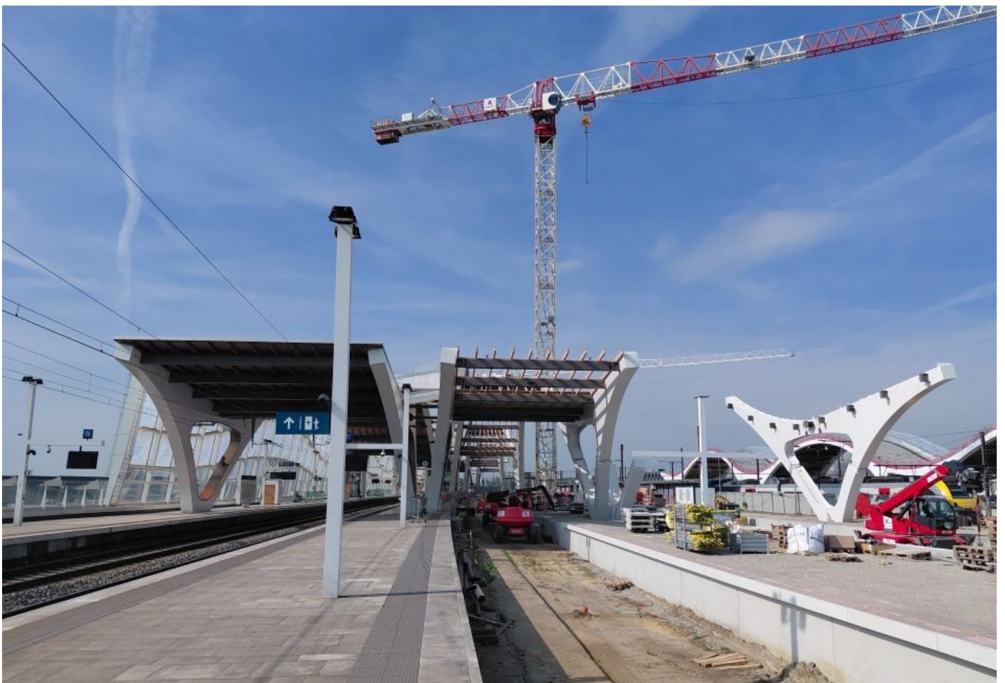
The original schedule for platforms were for them to open for the end of 2026 and looking at these photographs that may be possible. Photographs by Maxim Herman.
