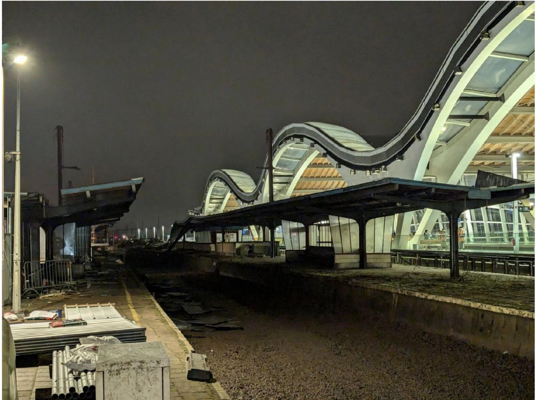
Demolition has started on Platforms 9 & 10 at Mechelen. A night shot by Nathan Van Riet - January 16th 2025
